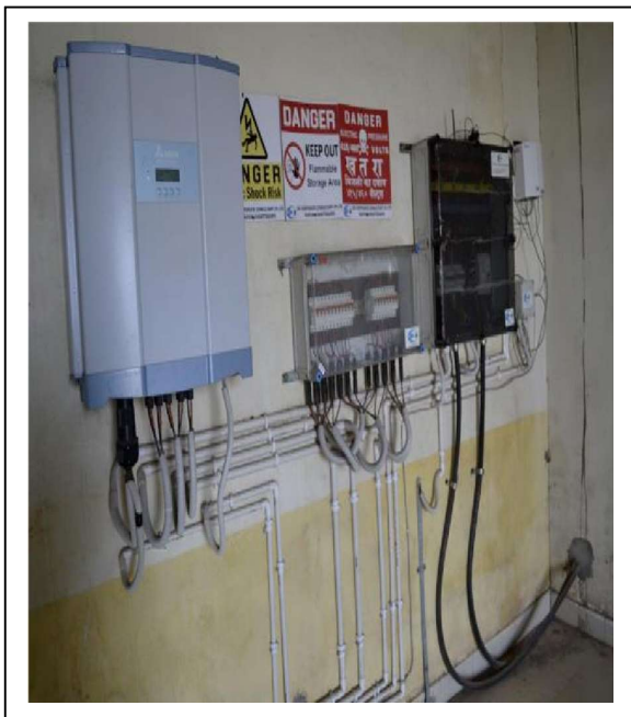
Solar control panel
